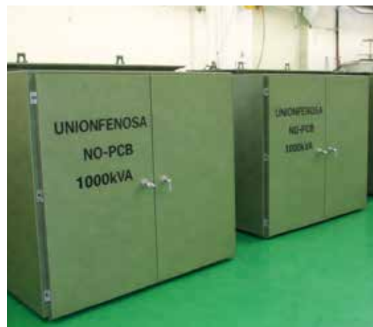
Pad Mounted Transformer 1MVA, Panama
