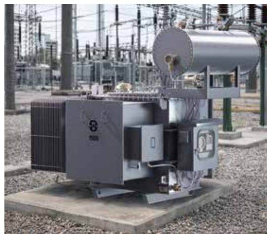
Distribution Transformer 2MVA, Hong Kong
